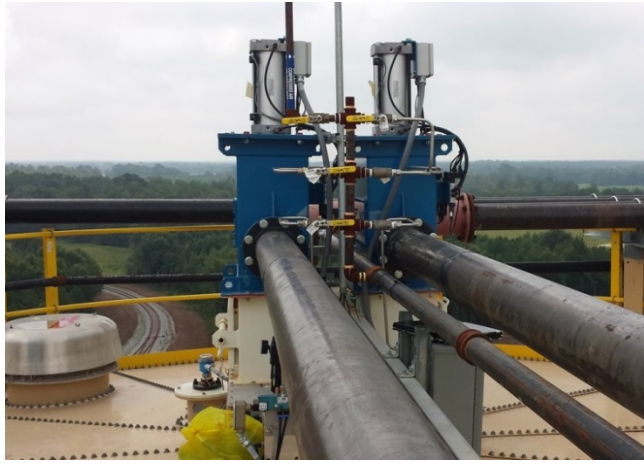
Diverter valves on the reception silo
